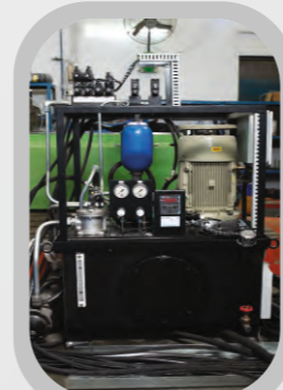
Hydraulic Power Pack
